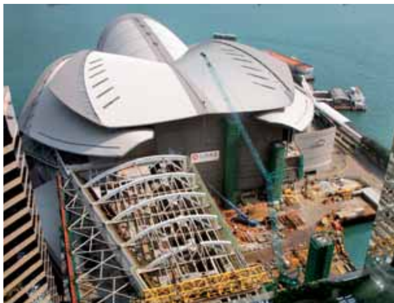
Expansion of Hong Kong Convention and Exhibition Centre Photo by Mr Cliff Wallace
